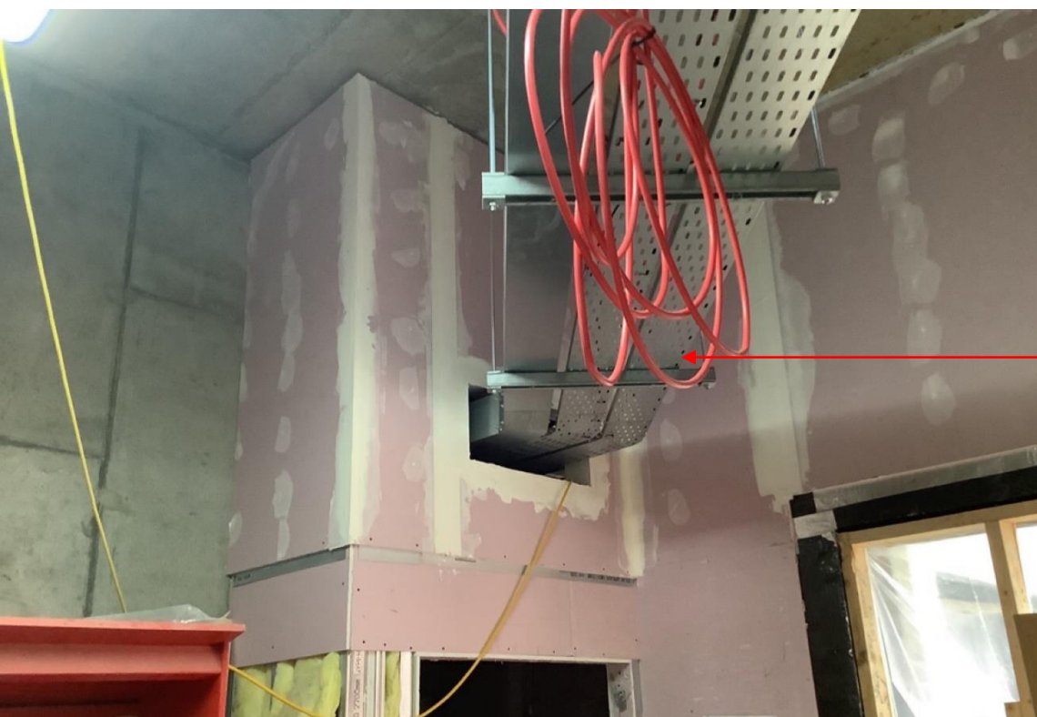
Services not serving the Firefighting Shaft passing through Fire Fighting Lift Lobby
