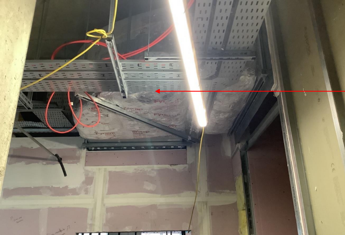
Services not serving the Firefighting Shaft passing through Fire Fighting Lift Lobby
